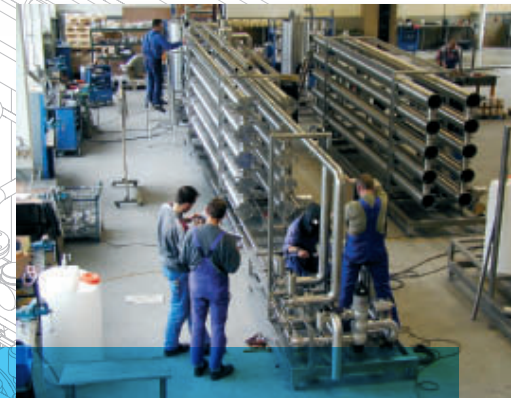
Anlagenaufbau einer Umkehrosmose- anlage 8" in Werkstoff 1.4404 (316L) 8" Reverse osmosis plant during construction, material: 1.4404 (316L)
